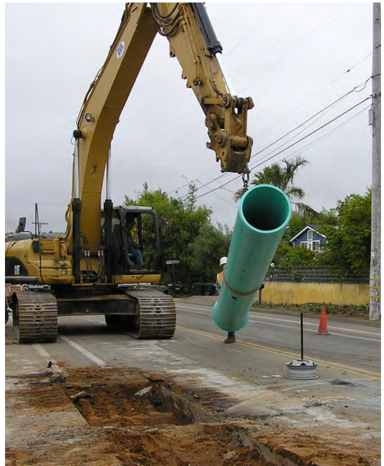
The Force Main Project Team lays down a 24" diameter PVC pipe along La Costa Avenue. Made of chemically stable polyvinyl chloride, the new pipeline will last 50+ years.
