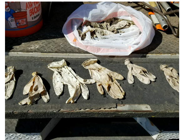
Rubber gloves found in the sewer pipes in Encinitas.
