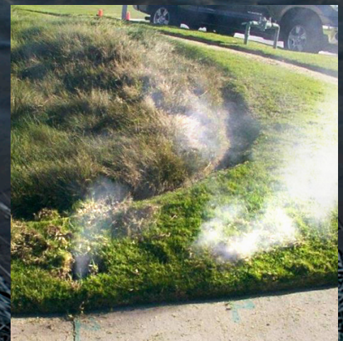
Smoke drifting from cracked pipes
