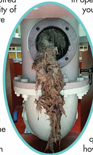
Recent blockage in District pump
