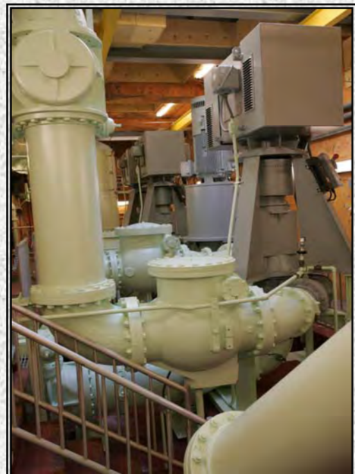
Batiquitos Pumping System
