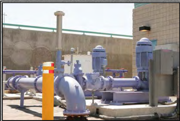
Recycled water facilities
