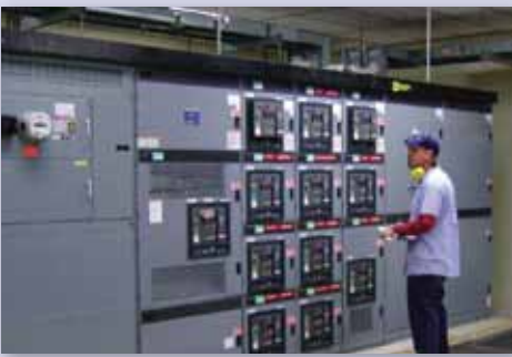
Operator Eric Have monitors the electrical activity at the plant.
