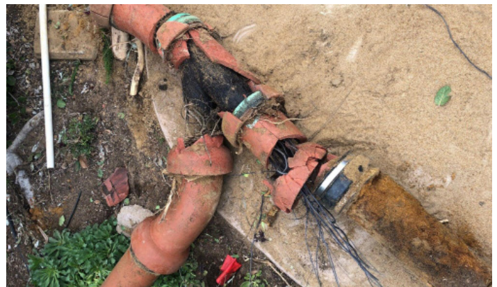
Large root inside Mr. Hooker's sewer lateral
