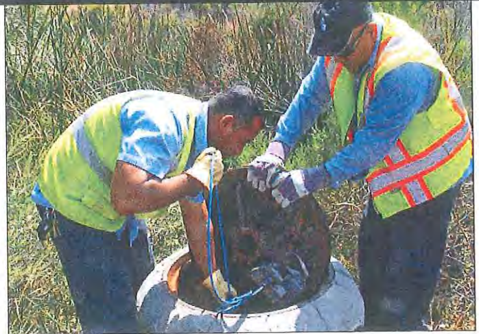
Field service technician Maurico Avalos, left, and field service supervisor Marvin Gonzalez install a SmartCover monitor from Hadronex.
