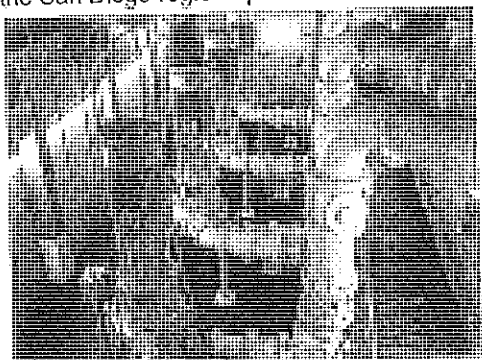
One of many sewer lift stations
