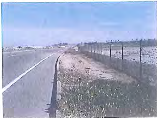
Location of force main break on Hwy 101.
