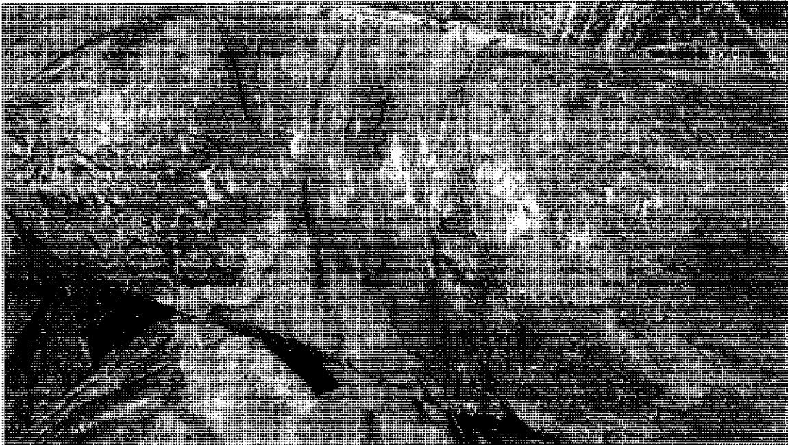
Heavy corrosion product build up on L1 Exterior (PE removed).
