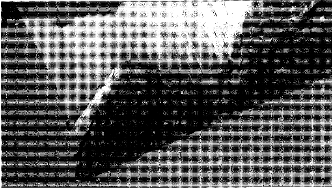
Arrows delineate internal corrosion initiating at edge of failed liner (liner removed during cleaning)
