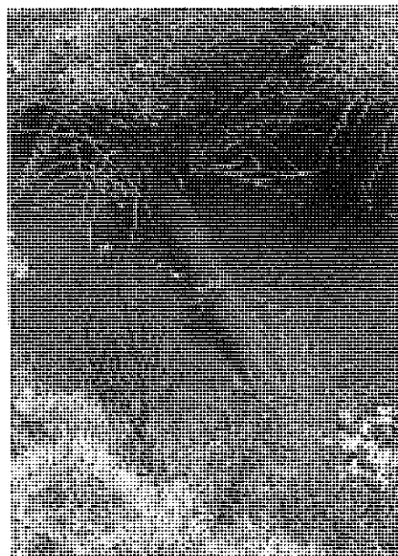
12" ACP exposed at creek crossing
