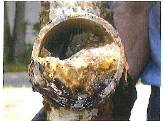
Wastewater pipe filled with FOG from residential and commercial buildings.
